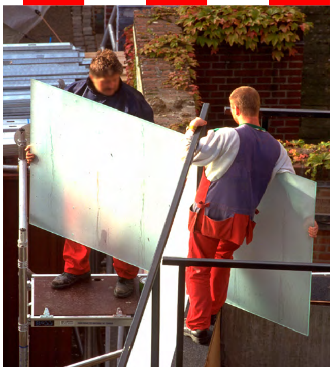
The worker has a high risk of falling, and the employees are not secured against falling
