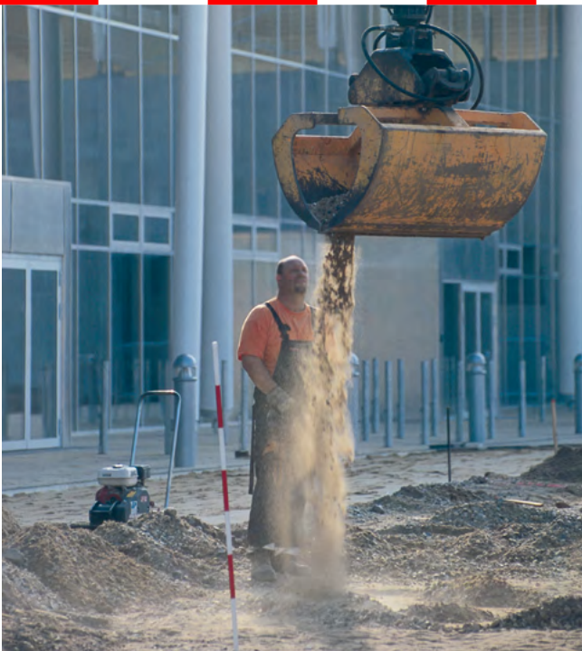
The worker is not using personal protective equipment and is too close to the moving parts of the machine; this comprises a high risk for accidents
