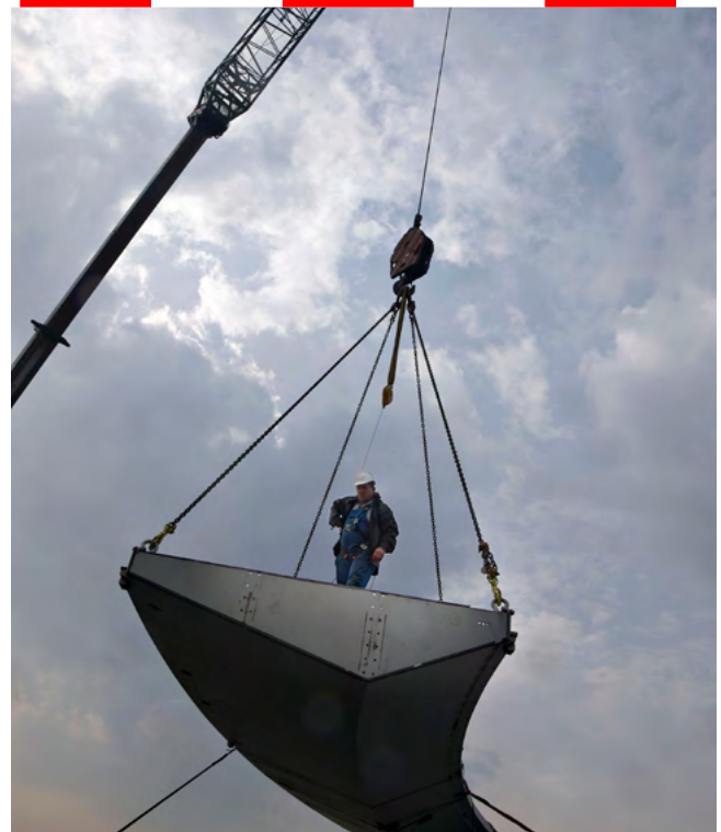
Unlawful securing of employees against falls
