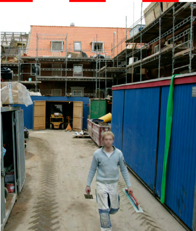
Not wearing a helmet at a construction site
