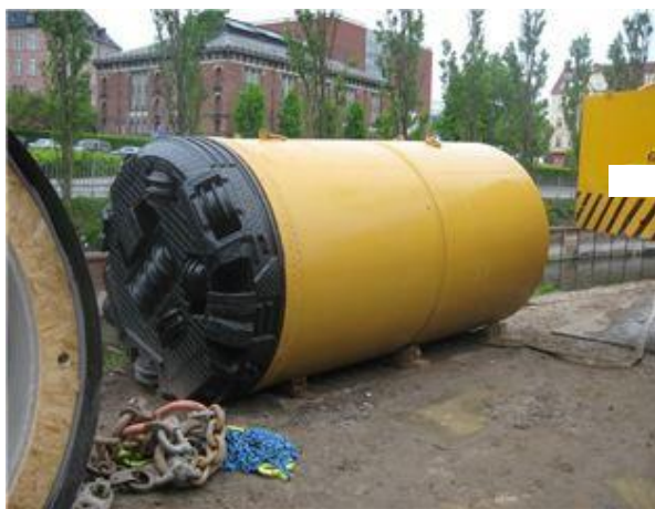
Borehoved for mikrotunneling - slurymaskine
