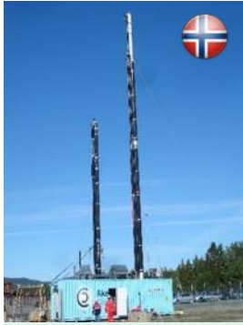
Natural gas Risavika Gas Center
