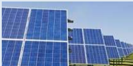
On-site solar park Schwarzheide, Germany
